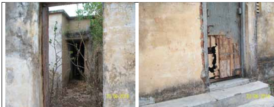
Staff quarters in dilapidated condition in PHC, Baravhi (Betul).
