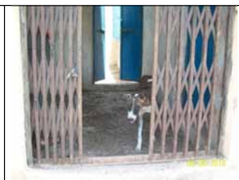
Building of SC Himmatgarh, (Dist: Dhar) lying unused, while it was functioning from another building.
